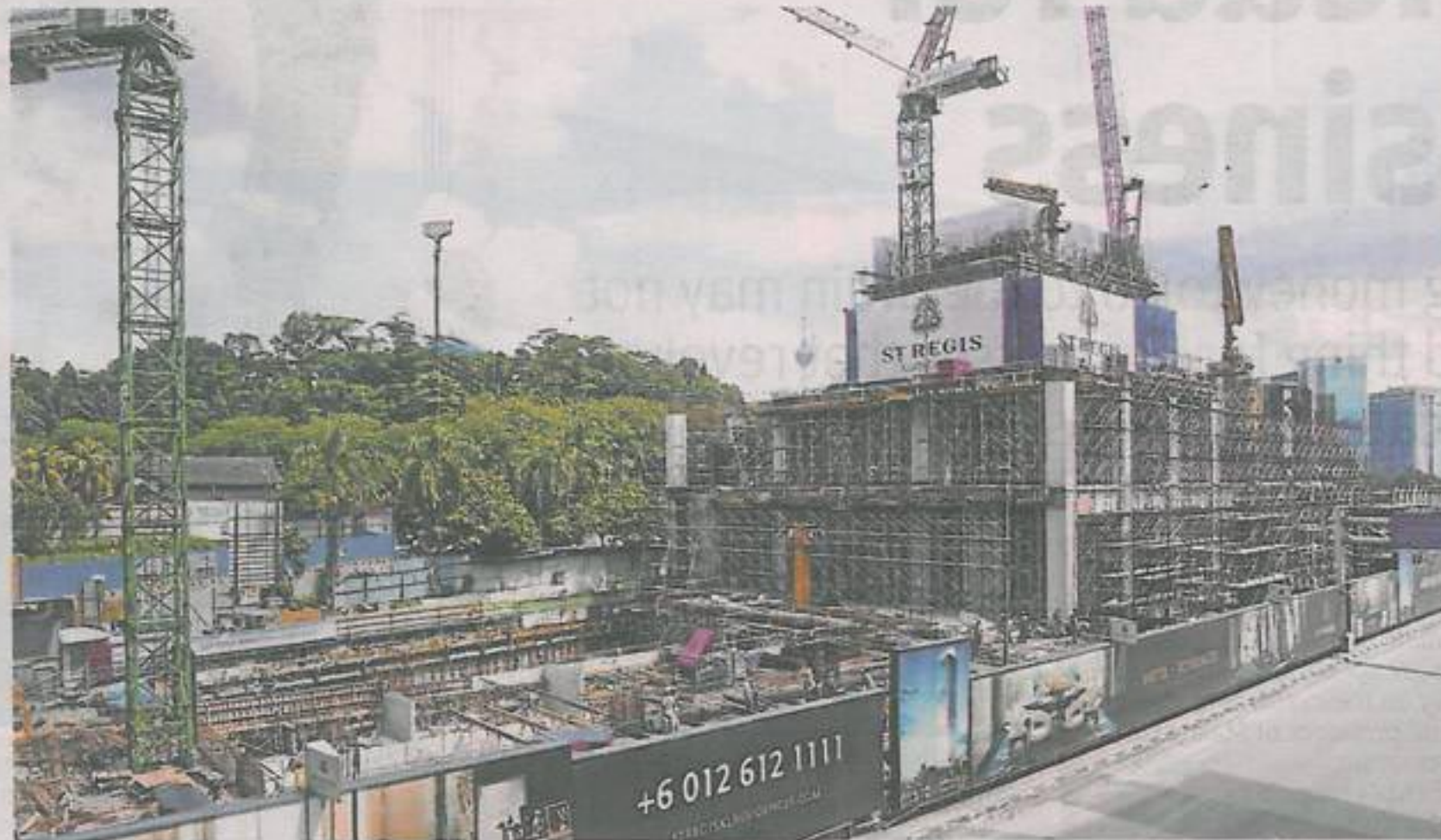
In progress: Work progressing at the St Regis site in KL Sentral, Kuala Lumpur. Construction is due to complete by December 2014.
